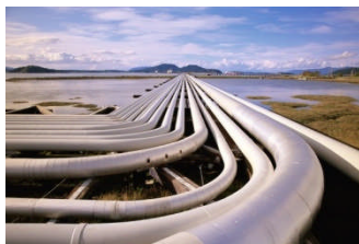
Natural Gas Pipeline
